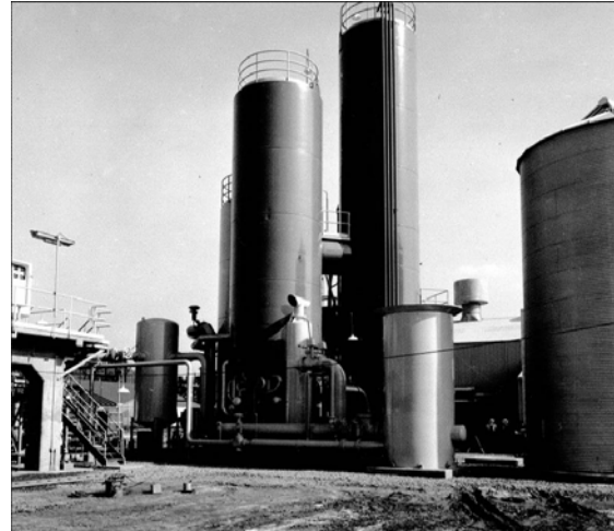
Figure 16b. Air separation plant of the early 1950s. 100 t/d. Photo courtesy Praxair.
